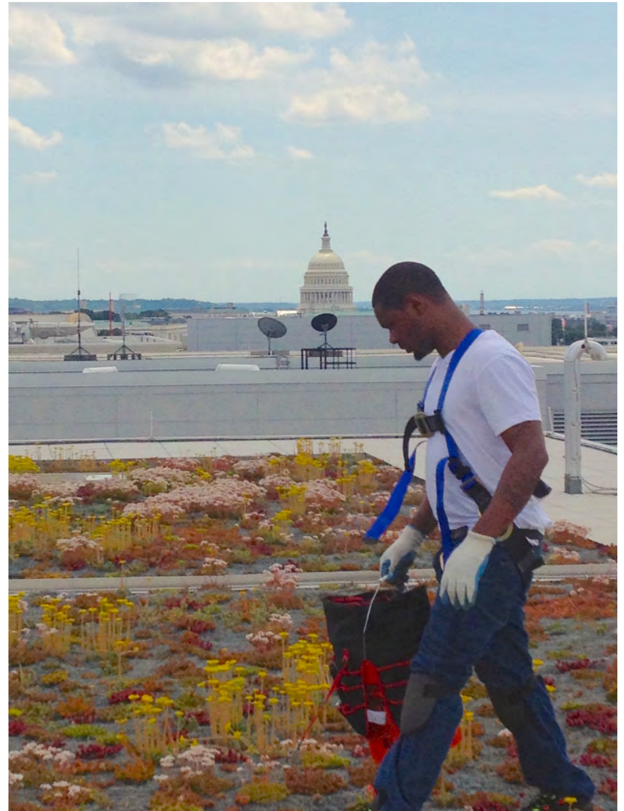
Photo 2. A D.C. Greenworks trainee performs maintenance on a green roof near the US Capitol Building. Photo credit: Neil Qusba at DC Green Works.
